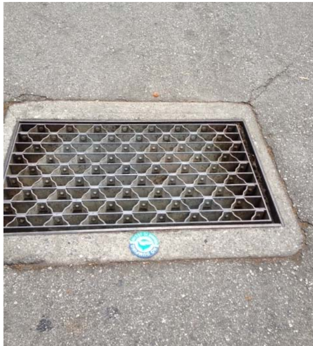
Photograph 12: Marked storm drain inlet in the parking area.
